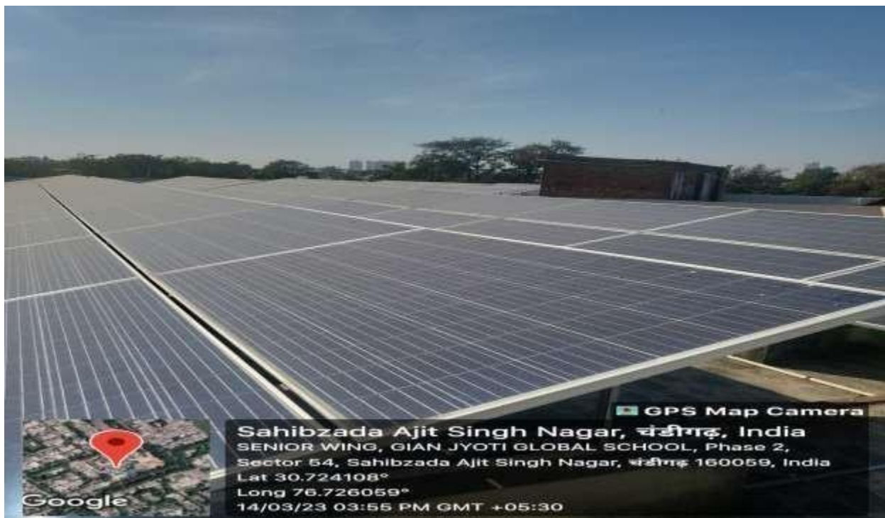
Solar Power plant (200 KWP) installed in campus
