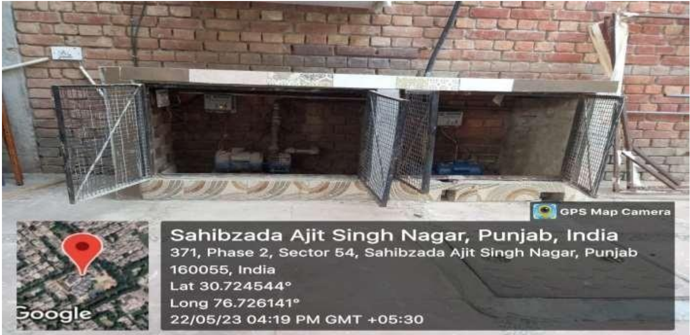
Motor – Pump sets transporting water from underground tanks to overhead water tanks
