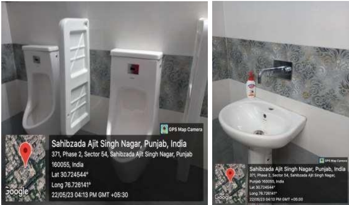
Fig: Automatic sensor-based Water urinals being used in building of GJIMT
