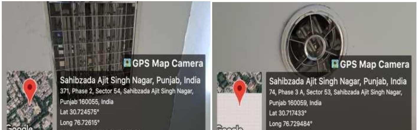
EXISTING 2 X 2 AND ROUND CFL FITTINGS IN CAMPUS
