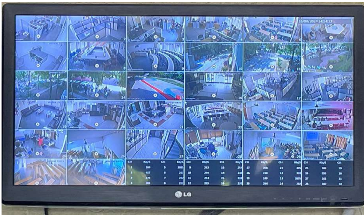
Fig: CCTV Surveillance View from the Director's Cabin, GJIMT.
