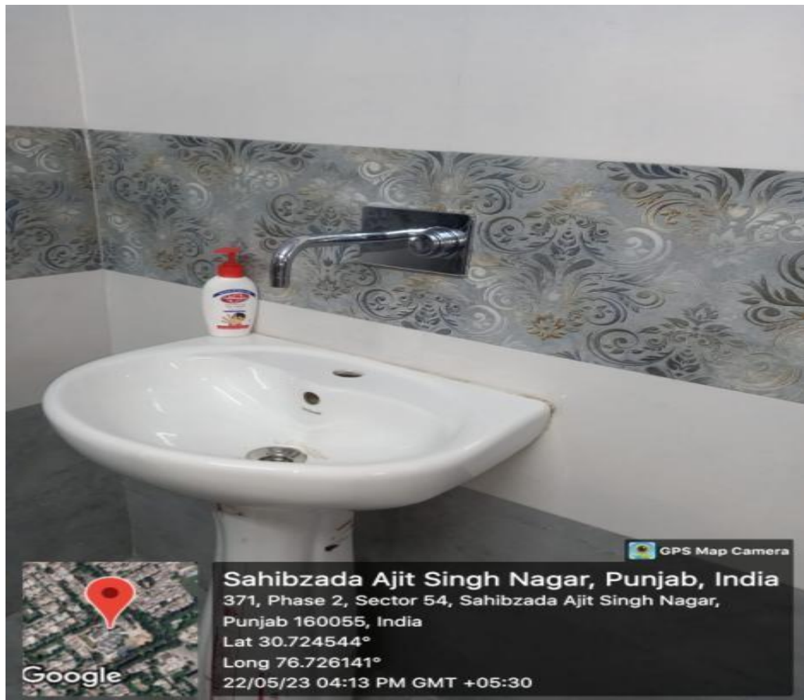
Pressmatic taps installed in Washroom
