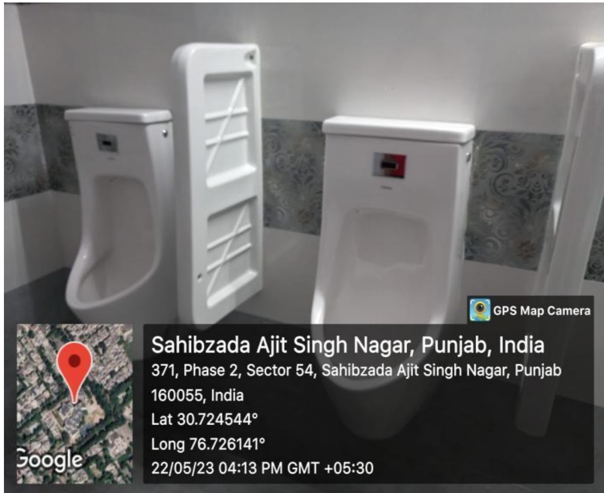
Urinal Sensor Flusher installed in Washroom
